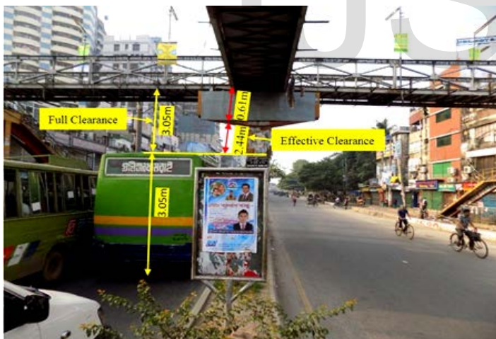
Fig 3: Reduced headroom due to hammer head pier (Science Lab Footbridge, Field Survey, 2015)
